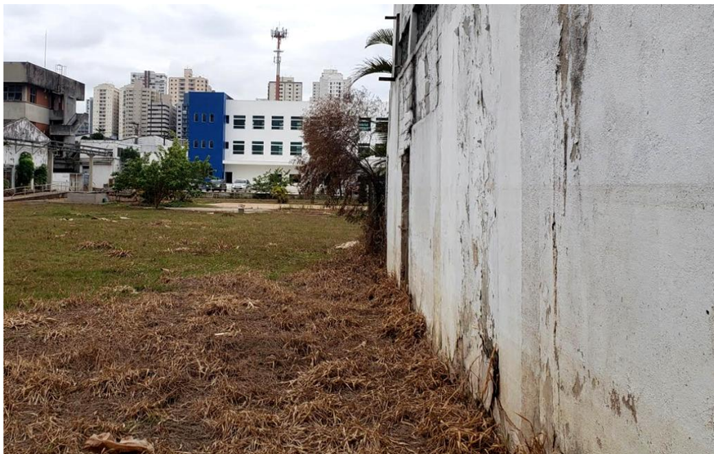
Figure 3 - Site after flooding event (March 2019) with water marks above 1m high on one of the former industry walls. In the uphill background are recent commercial and residential buildings.
