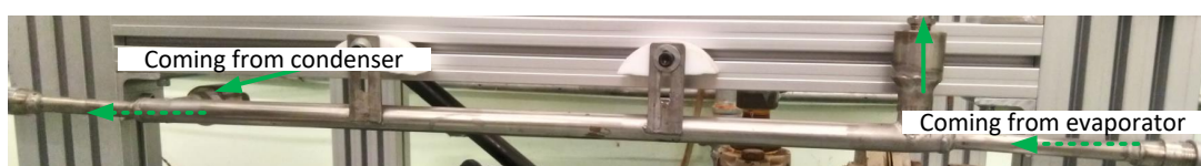
Figure 5.8 – Subcooler for ammonia liquid subcooling
