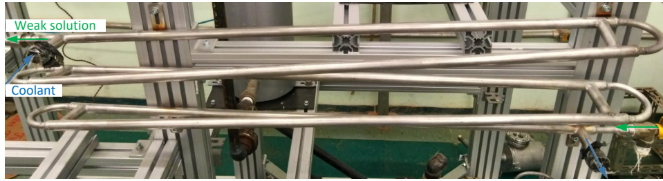
Figure 5.14 – Still picture of the subcooler for weak solution temperature control
