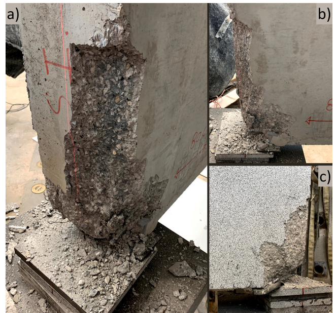
Fig. 16. Right support region after the test.
