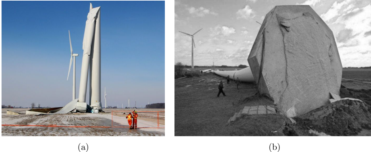
Figure 2: Examples of structural damage in wind turbine systems due to structural design failure: (a) structural tower collapse (Shreve, 2018) [1] and (b) collapsed structure due to cracks in the foundation (Fowler, 2021) [2].
