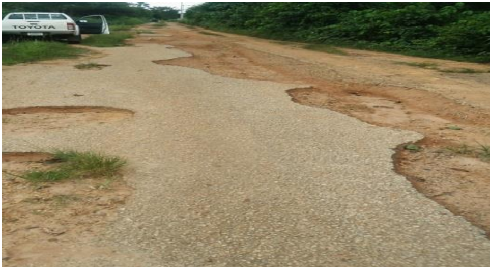
Figure 23 - Road condition from Mulekangbo to Ilubirin community
