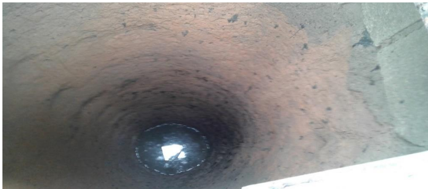
Figure 31 - Bitumen seepage in hand-dug well
