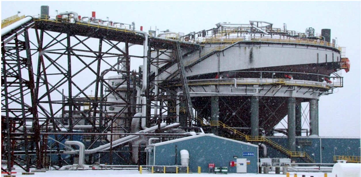
Figure 17 - View of sloped inlet piping feeding into a PSC
