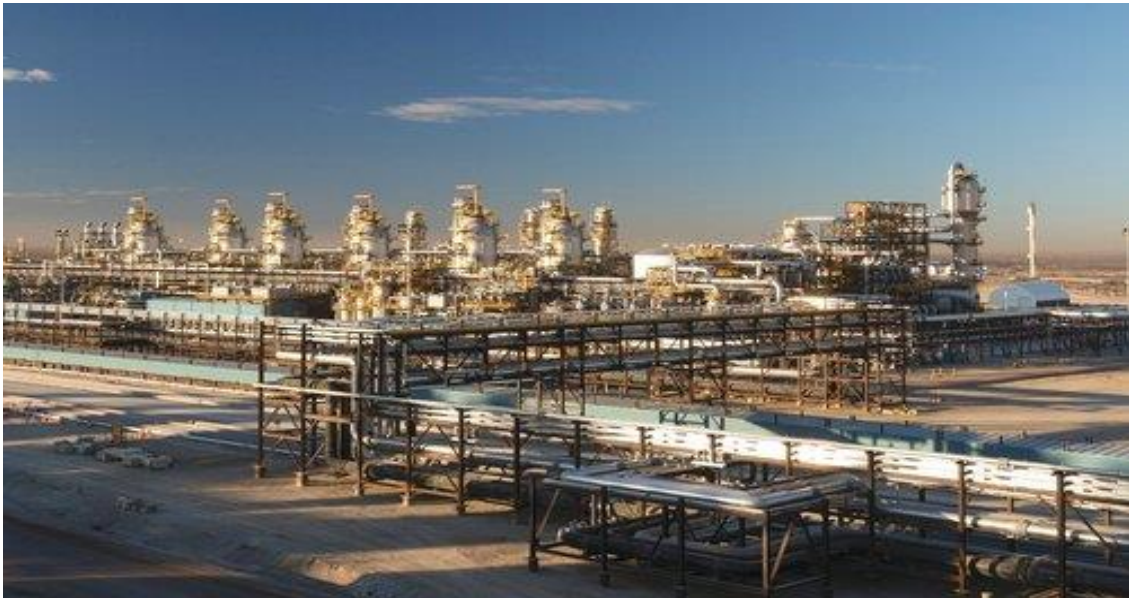
Figure 18 - Froth treatment unit
