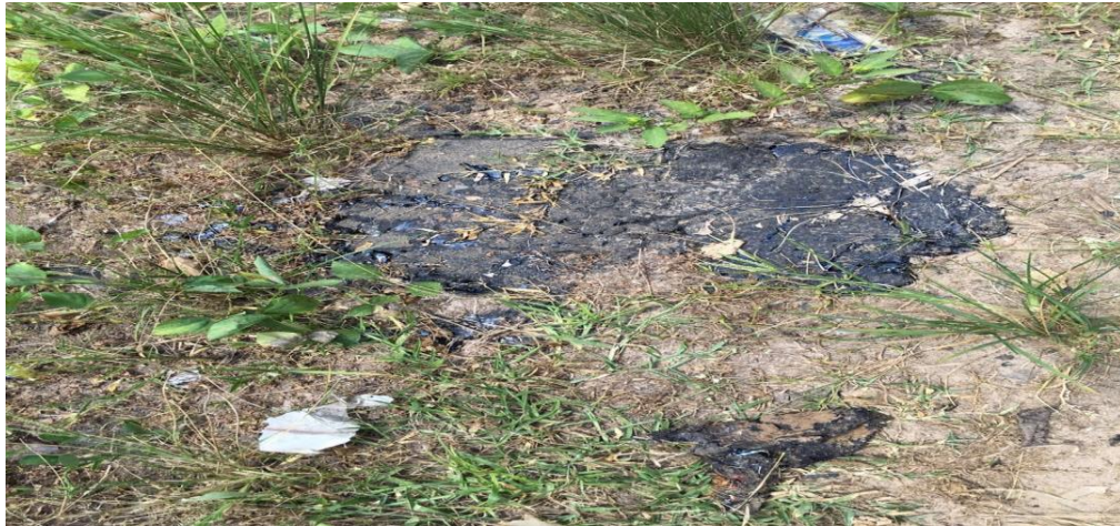
Figure 24 - Bitumen seepage in Ilubirin community
