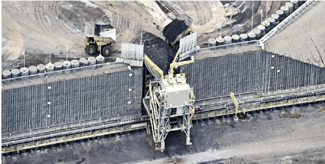
Figure 15 - Truck dumping mined oil sands into the top of a crusher installed within a retaining wall. Photo courtesy Shell Canada.
