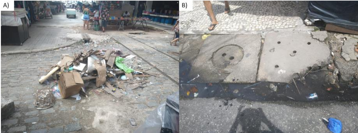
Figure 17: Photographic records of the study area. A) debris left by merchants; B) example of a damaged curb drain.
