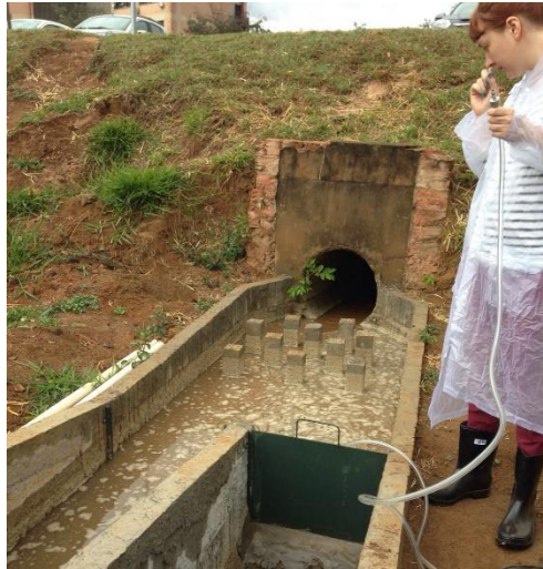
Figure 3.6 – Example of bioretention applied in the outlet of conventional drainage system, for an application in street scale catchment
