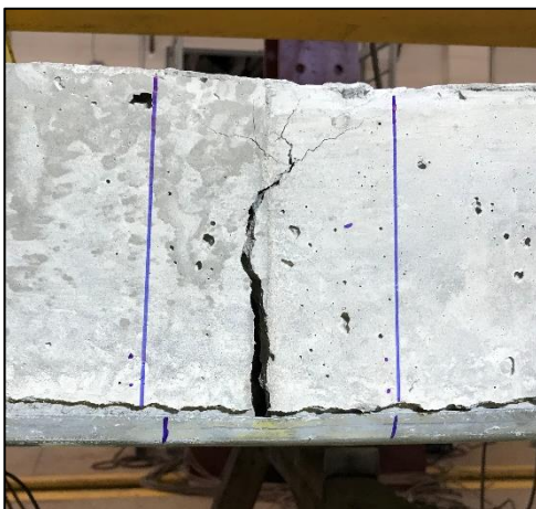
(a) Fissura principal
