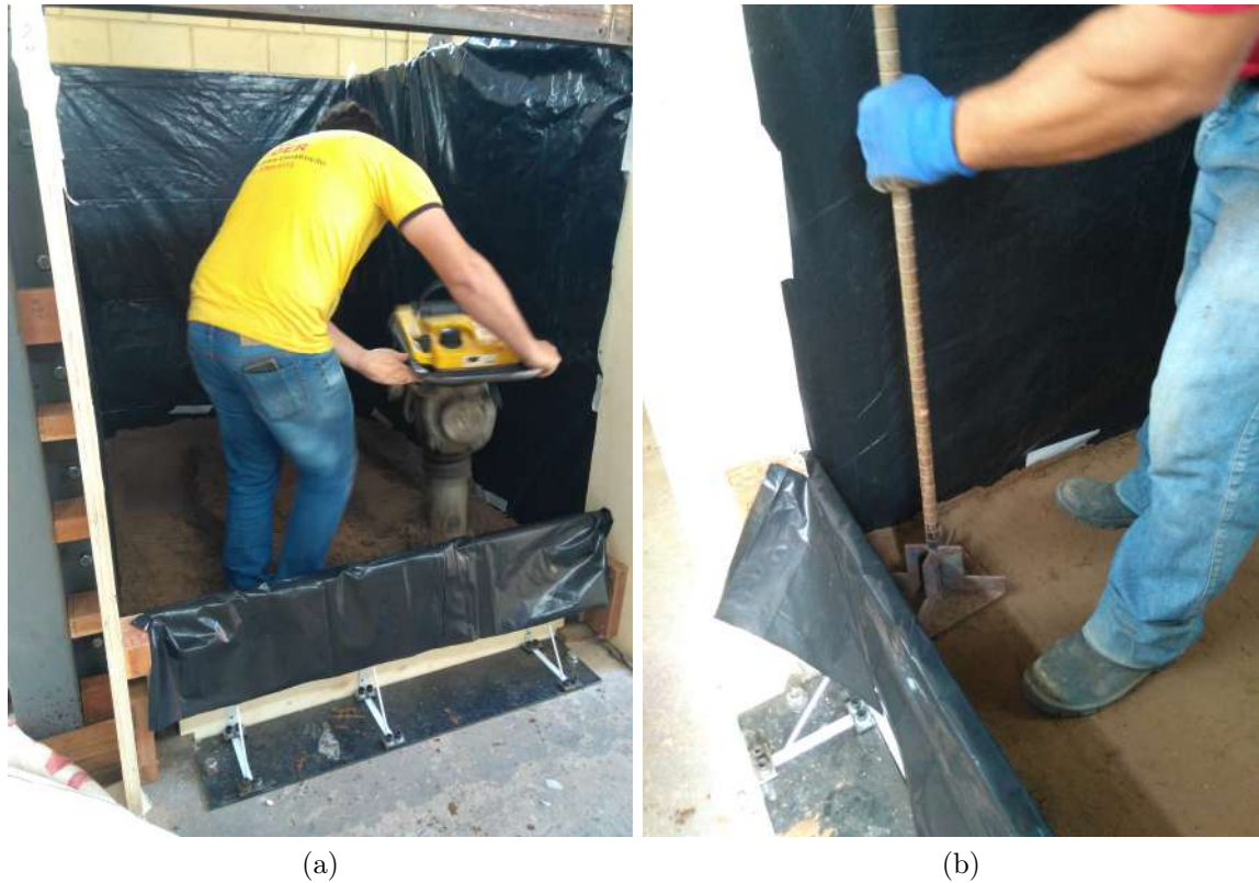
Figure 5.62: Foundation compaction: (a) hand operated compactor; (b) manual compactor for final adjustments.
