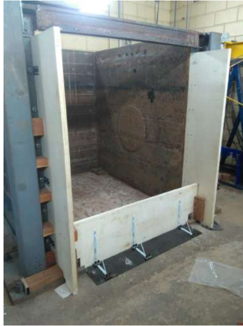
Figure 5.17: Lateral plywood sheets installed to provide lateral support for the modular block facing and temporary frontal plywood sheet to provide confinement for the compaction of the foundation soil.
