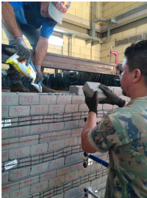
Figure 5.64: Detail of instant grout used to glue together the top three rows of block.
