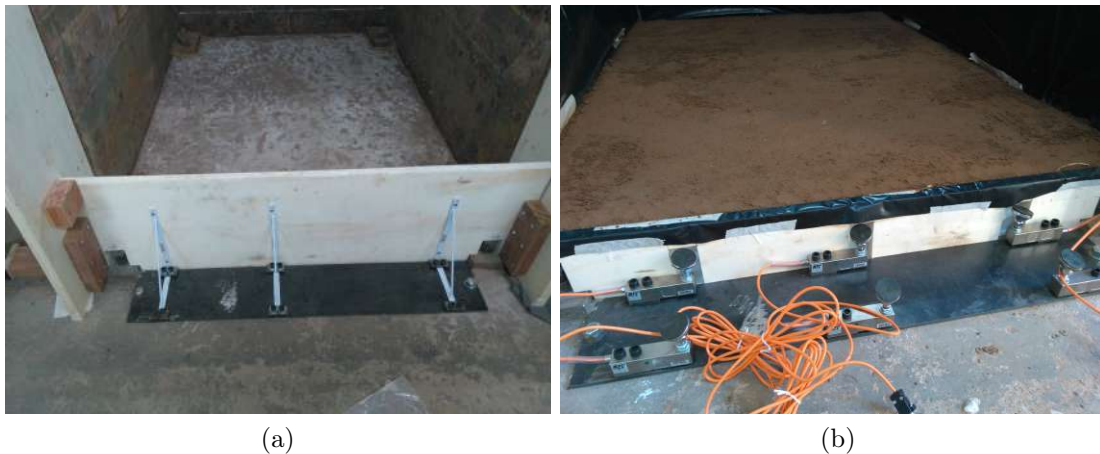
Figure 5.61: Test box front foundation support (a) temporary support for soil foundation compaction (400 mm high); (b) permanent support (160 mm high).
