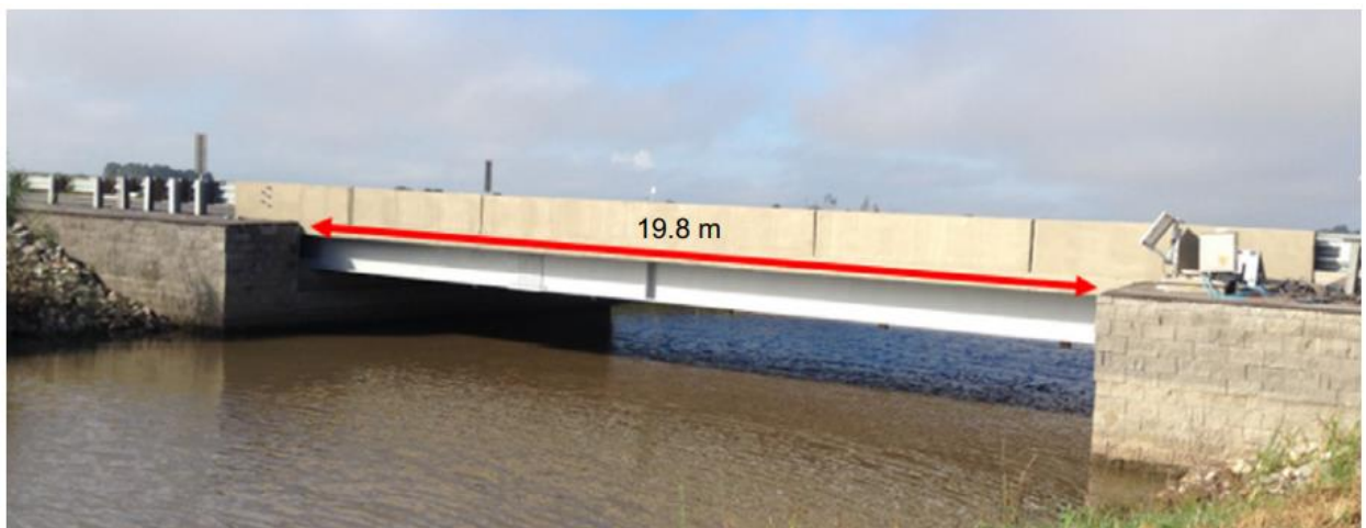
Figura 5. Ponte GRS-IBS Maree Michel (Ardah et al. , 2018).
