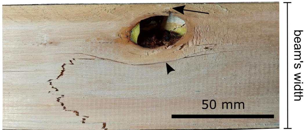
Figure 32. Knot on the tensioned side of beam 18 which caused an early rupture. The arrow points the rupture on the thin knot edge and the arrow head points the rupture in the transition between wound wood and regular wood.
