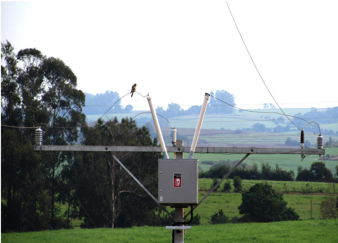
Figure 2.9. Voltage measuring system (pole PX2) [52].
