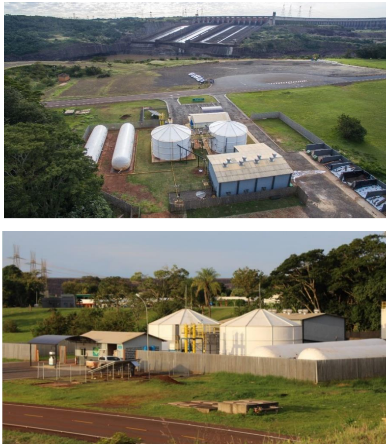
Figure 6: Itaipu Production Unit. Source: CIBiogas files
