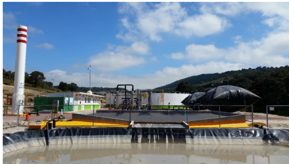
Figure 21: Waste treatment plant in Atacomulco, México. Source: AMBB files.
